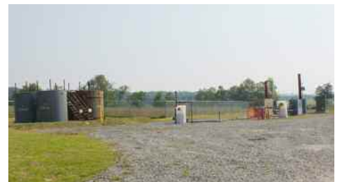
Cabot operational well site, with the rig removed and surrounding land reclaimed. Photo: Laurie Stephens
